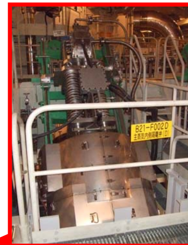
主蒸気隔離弁(8台)
