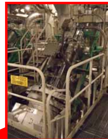
主蒸気隔離弁(8台)
