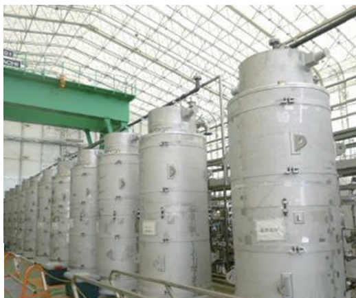
High-performance multi-nuclide removal equipment (absorption towers)
