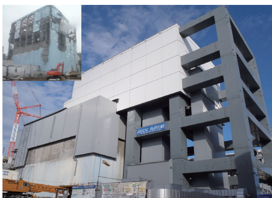
The extended structure and covering installed onto Unit 4 reactor building for the removal of fuel (Left above: Unit 4 reactor building immediately after the nuclear accident in March 2011)
