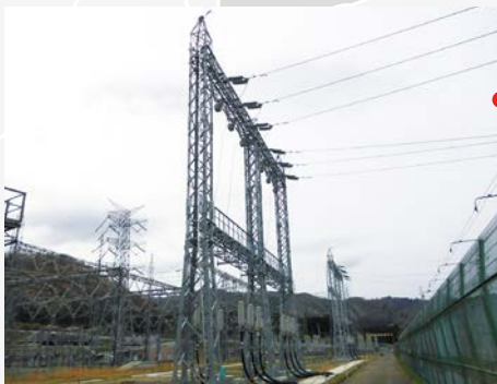
New Fukushima Substation
