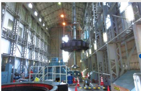
Nippashigawa Hydro Power Station
