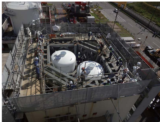
Installing iodine filters as part of above-ground filtered vent equipment of the Kashiwazaki-Kariwa Nuclear Power Station Unit 7
