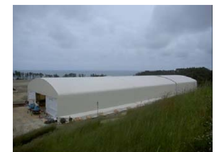
Fig. 5: Preparation work for covered temporary storage facility preparation completed (first building, taken on June 13, 2012)
