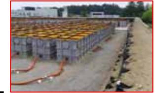
Square shape steel tanks (desalinated water, RO waste water)
