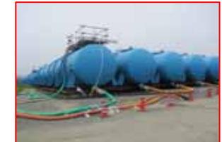
Lying steel tanks (evaporative concentration water tanks)
