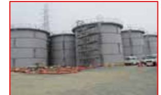
Round shape steel tanks (desalinated water, RO waste water)
