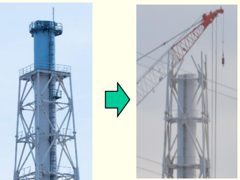
Before dismantling / Dismantling of the 5th block was completed / Progress status in dismantling of the exhaust stack
