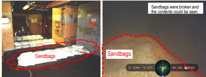
Condition immediately after the earthquake / Current condition of Zeolite sandbags
