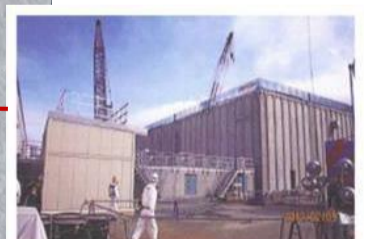
Temporary waste sludge storage
