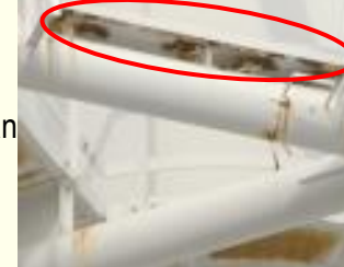
Potentially degraded scaffold material
