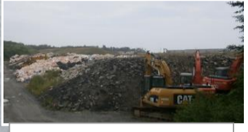
Rubble (outdoor accumulation)
