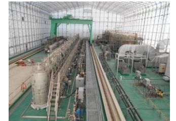
High-performance (multi-nuclide removal equipment)
