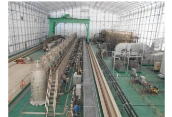
High-performance (multi-nuclide removal equipment)
