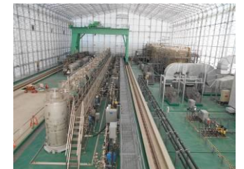
High-performance (multi-nuclide removal equipment)
