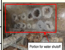
Water shutoff status at the penetration of Unit 2 intake power supply cable
