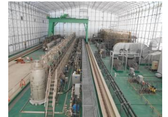
High-performance (multi-nuclide removal equipment)
