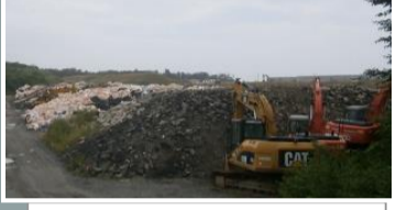
Rubble (outdoor accumulation)
