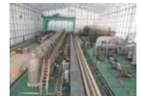
(High-performance multi-nuclide removal equipment)
