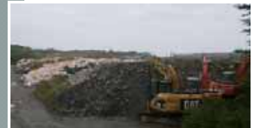
Rubble (outdoor accumulation)
