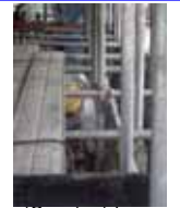
(Opening/closure of frozen pipes)
