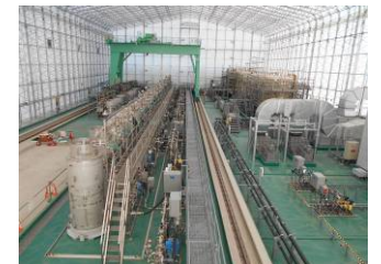
(High-performance multi-nuclide removal equipment)
