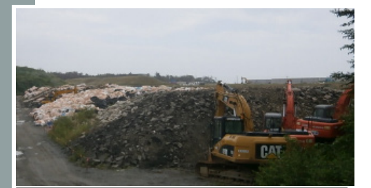
Rubble (outdoor accumulation)
