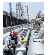
(Opening/closure of frozen pipes)
