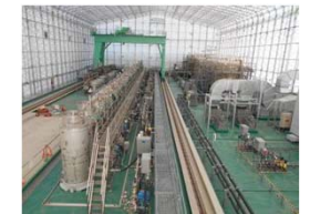
(High-performance multi-nuclide removal equipment)
