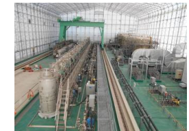
(High-performance multi-nuclide removal equipment)
