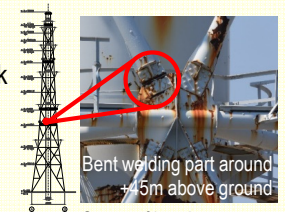
<Status of breakage>
