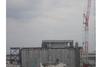
Installation of a cover for fuel removal at Unit 3 Installation of reinforced members for FHM girder
