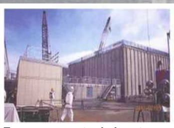
Temporary waste sludge storage
