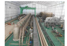
(High-performance multi-nuclide removal equipment)
