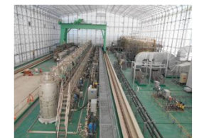
(High-performance multi-nuclide removal equipment)
