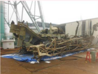
Fuel handling machine removed from the pool
