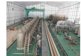
(High-performance multi-nuclide removal equipment)
