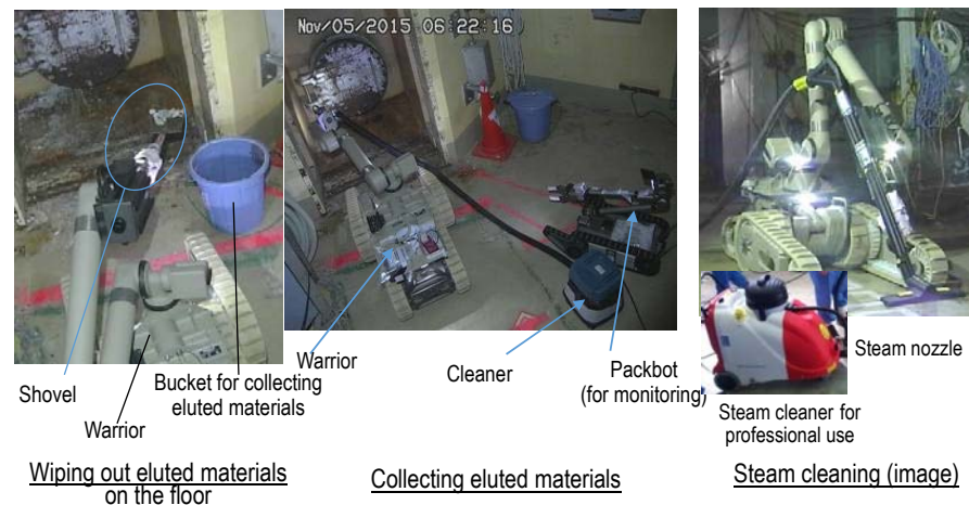
Figure 5: Decontamination around Unit 2 X-6 penetration
