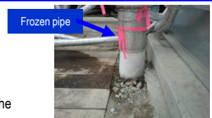
(Land-side impermeable walls; example of freezing functioning test point)
