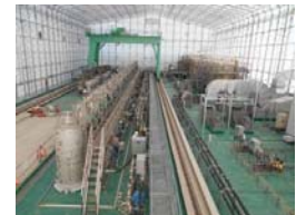
(Installation status of high-performance multi-nuclide removal equipment)
