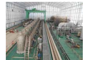
(Installation status of high-performance multi-nuclide removal equipment)
