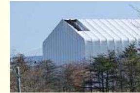
<Status of tent damage>
