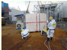
<Installation status of measurement equipment>
