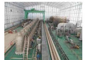
(Installation status of high-performance multi-nuclide removal equipment)
