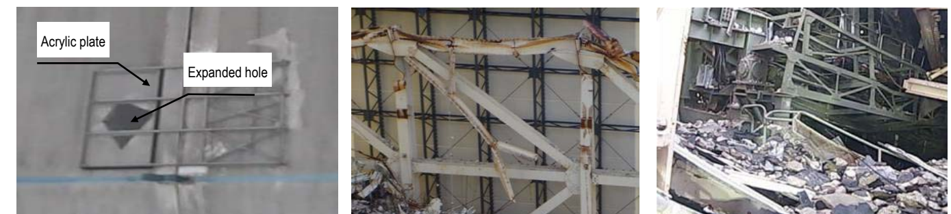
Covering status of expanded hole in roof panel of building cover Existing steel frame at upper part of Reactor Building Underside of collapsed roof
