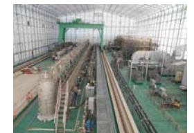
(Installation status of high-performance multi-nuclide removal equipment)
