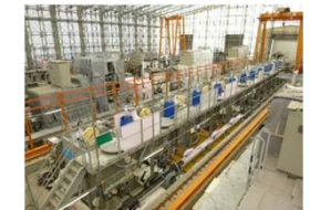
(Installation status of the facility to absorb radioactive materials)
