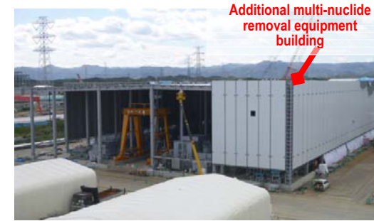
Figure 4: Overview of additional multi-nuclide removal equipment
