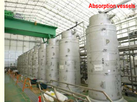
<Installation status of high-performance multi-nuclide removal equipment>
