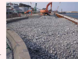
Installation status of impermeable walls on the sea side (Landfill status on the Unit 1 intake side)
