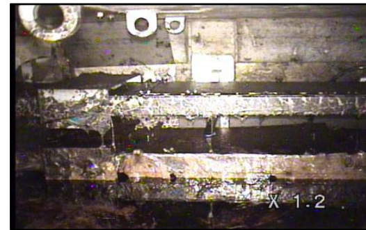
① Cable tray (above the water surface)
