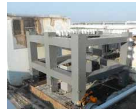
3. The second layer of the steel frame completed (Photo taken on February 28)
