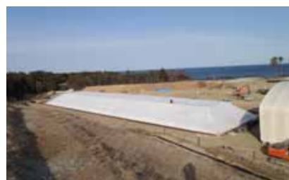
7. Current progress status of the second soil-covered type temporary debris storage facility (Photo taken on February 26)
