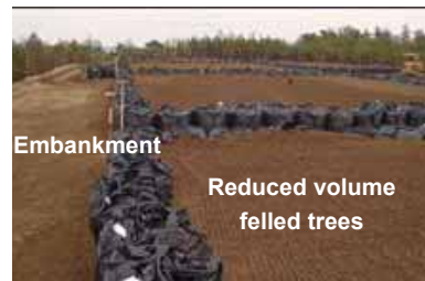
8. Current progress status of the temporary storage facility for felled trees (Photo taken on February 19)
