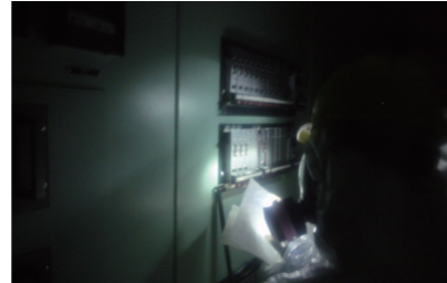
Connecting collected batteries to meters and gauges (main control room for Units 1 and 2)
