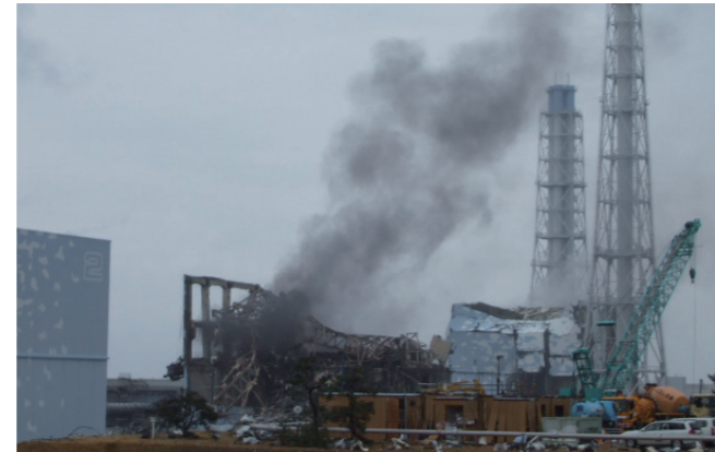
Unit 3 reactor building after the hydrogen explosion
