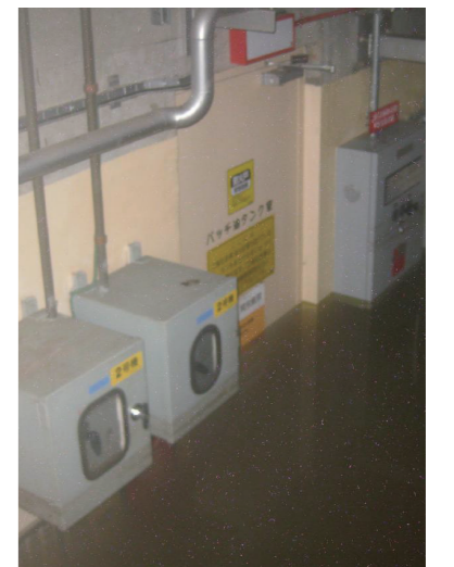
Flooded power room (Fukushima Daiichi Nuclear Power Station Unit 2)
