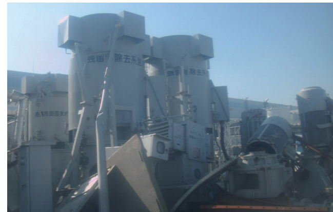
Seawater system pump that lost availability in the tsunami
