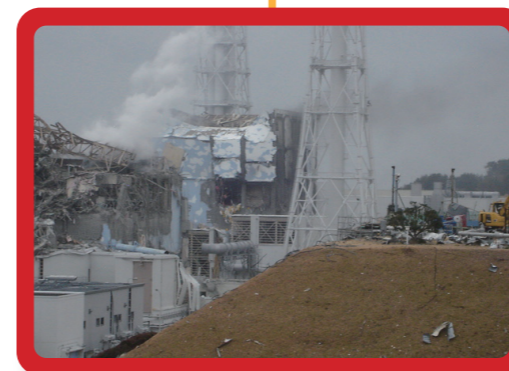
Around 6:14 a.m. Hydrogen explosion in the Unit 4 reactor building
