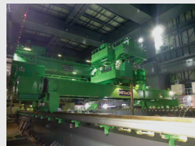
Overhead crane / fuel handling machine
