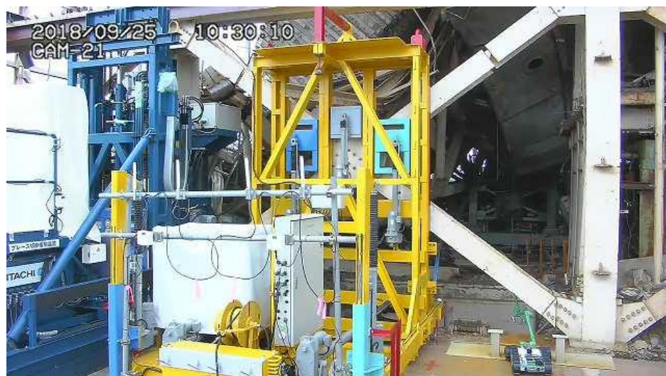
Bandsaw being used to cut off the X brace while a gripper is holding it
