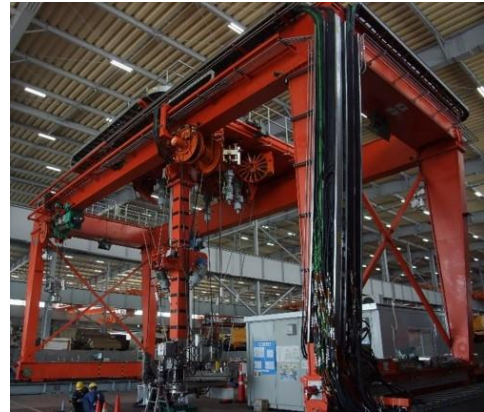
Unit 3 Fuel Handling Machine
