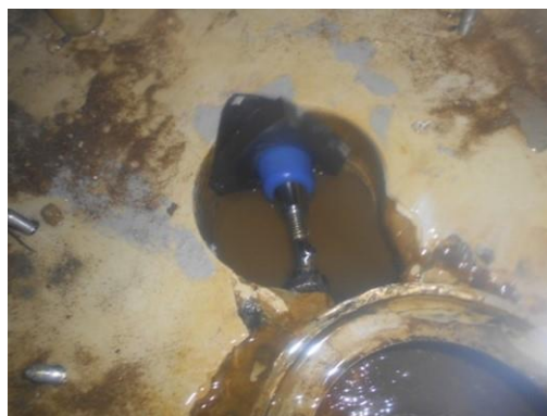
Hole temporarily plugged to stop water flow
