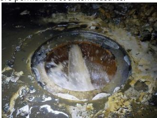
Floor funnel from which gushing water was found
