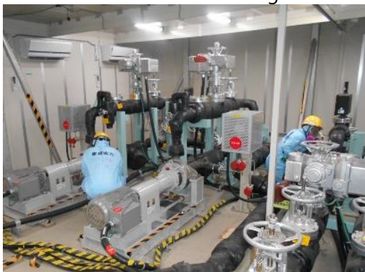
Field check of reactor coolant injection systems
