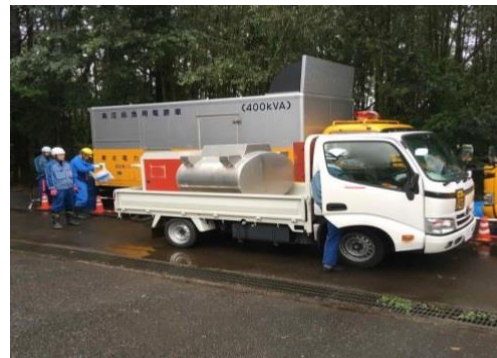
Filling a power supply truck with gasoline using a tanker truck from Fukushima Daini
