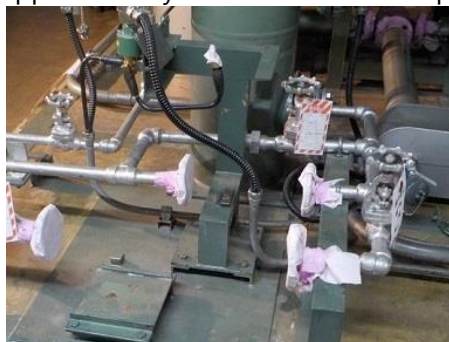
Prior to kaizen: Covered with fire-proof sheet
