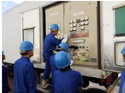
Sampling data prior to trial operation of replaced generator
