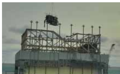
Start of rubble removal from top floor of Unit 1 reactor building (Jan. 22)
