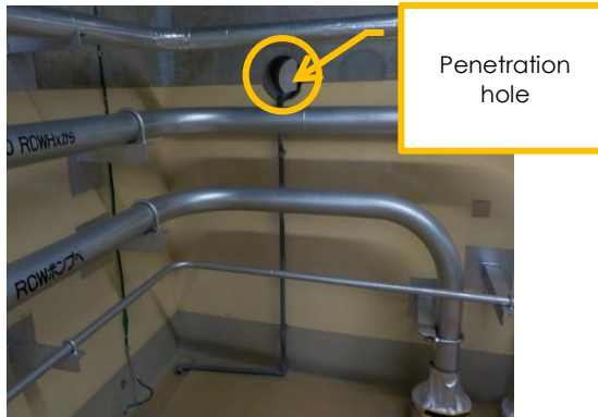
Penetration hole in a firewall that has yet to be fireproofed (Unit 2 reactor building subfloor 1)
