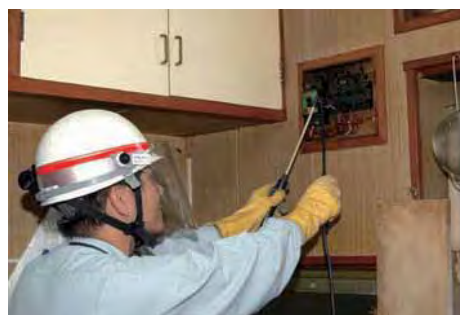
Wiring diagnosis for fire prevention (photo provided by Gakunan Asahi Newspaper)
