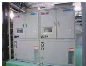
Heat pumps installed in Sony Energy Devices Corporation
