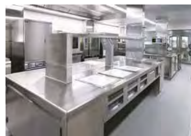
Industrial electrified kitchen
