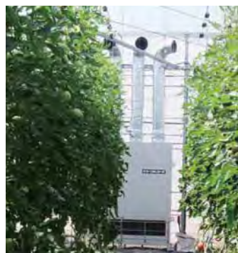
Heat pump for gardening purpose installed in a tomato greenhouse
