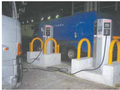
Power supply system introduced to Tsukiji Market
