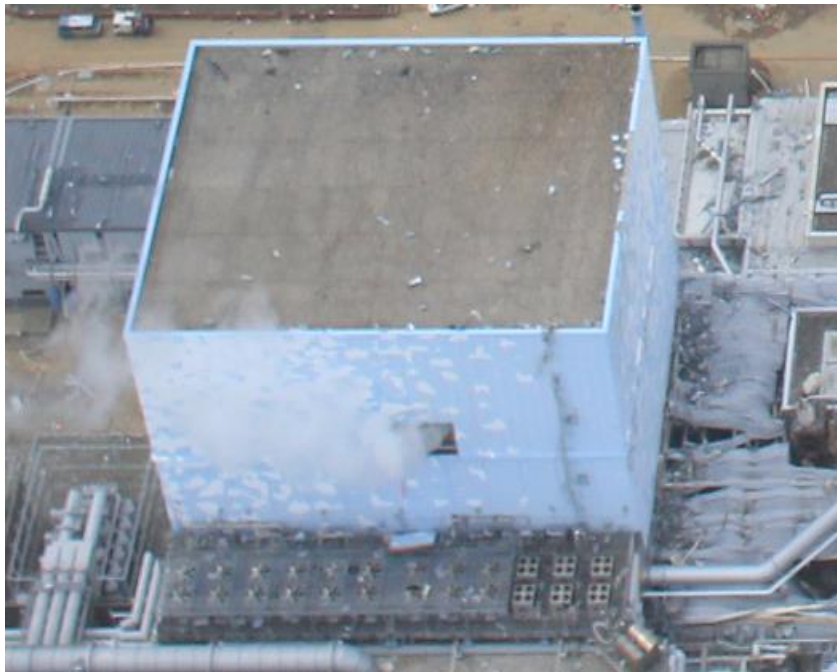
Figure Opened blow-out panel of Unit-2
