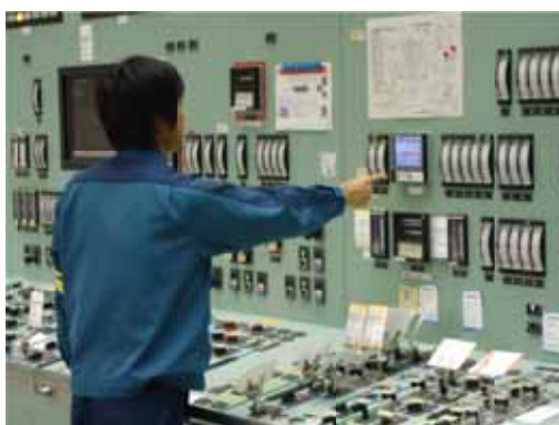
Monitoring of spent fuel pool water levels in the main control room (front panel)
