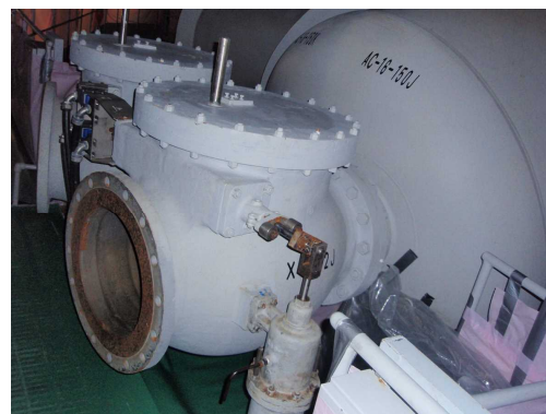
Figure 2 Vacuum breaker valve
