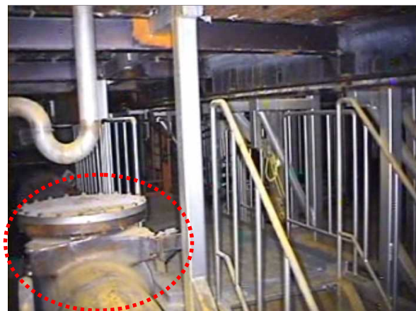
Figure 2-3 Camera photo of an S/C vacuum breaker in the torus room of Unit-1
