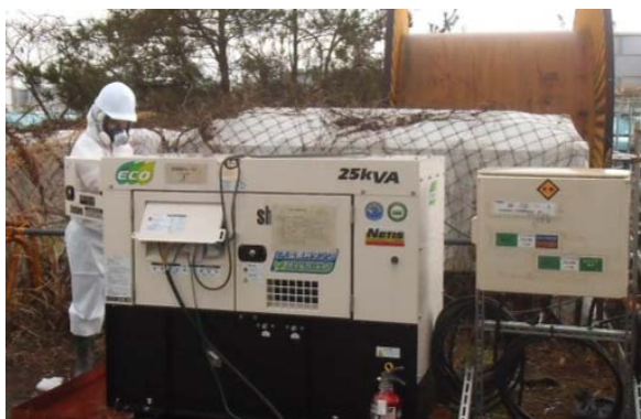
Connection and operation drill of temporary power generator (Fukushima Daiichi)
