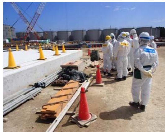
On-site safety control instruction being provided to TEPCO/prime contractor employees by an independent expert
