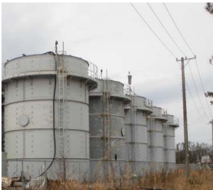
Improvement-2: Flange type tanks before improvement
