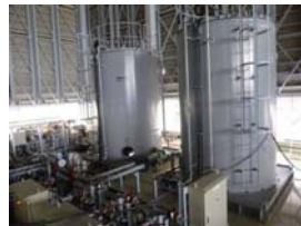
Increased number of ALPS (Contaminated water receiving tank)
