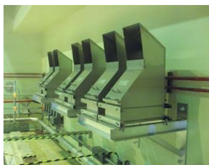
Unit 6 Reactor building hydrogen processing system
