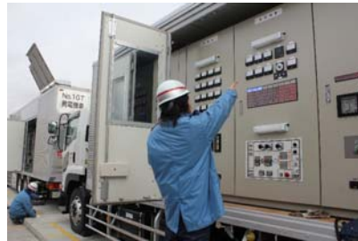
Actuation operation of gas turbine generator vehicle
